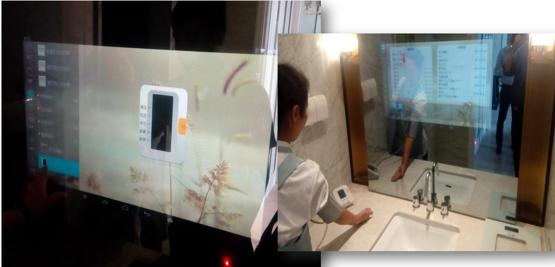
Above: Newly installed innovative smart home system
